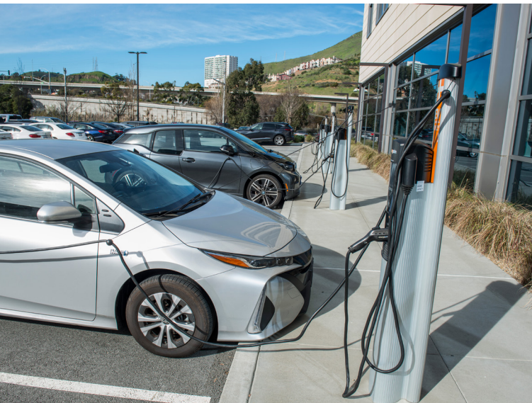
Electric Vehicle Charging
