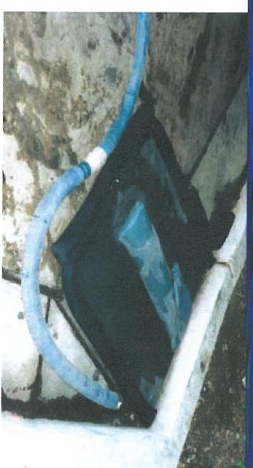
A storm drain cover with a vacuum hose.
