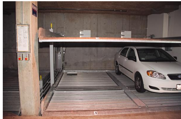
Figure 4-7: Parking Lifts in Parking Garage, Berkeley (Courtesy of City of Berkeley)
