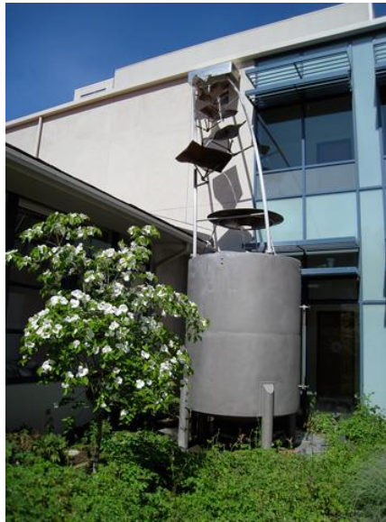
Figure 8-10: Rainwater Harvesting Cistern in Oakland at Mills College (Credit EOA, Inc.)
