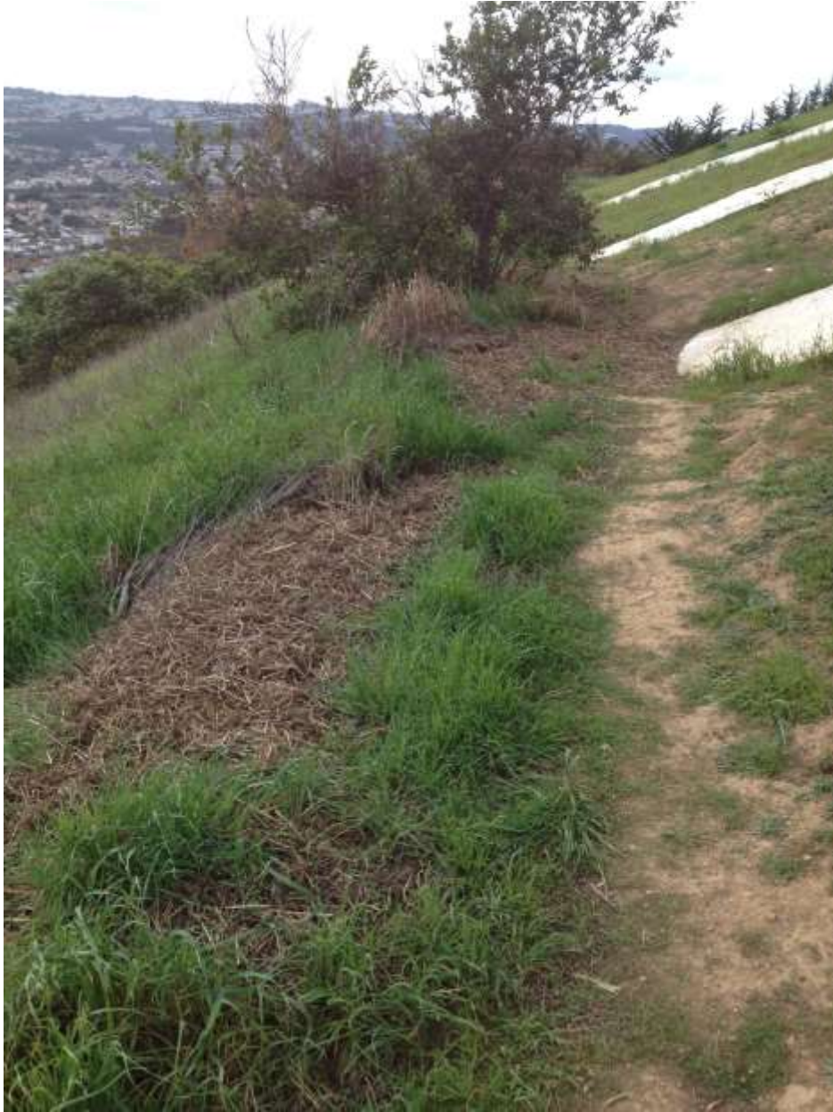
View 6. View of debris piles from treated slopes along the base of the historic sign, where current practices appear to involve raking slash rather than leaving it in place which would be more desirable to build up thatch necessary to help control establishment and spread of invasive groundcover species and to improve habitat conditions.
