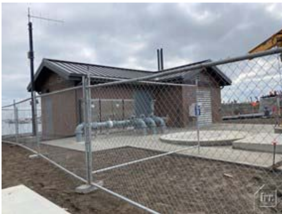
Sewer Pump Station
