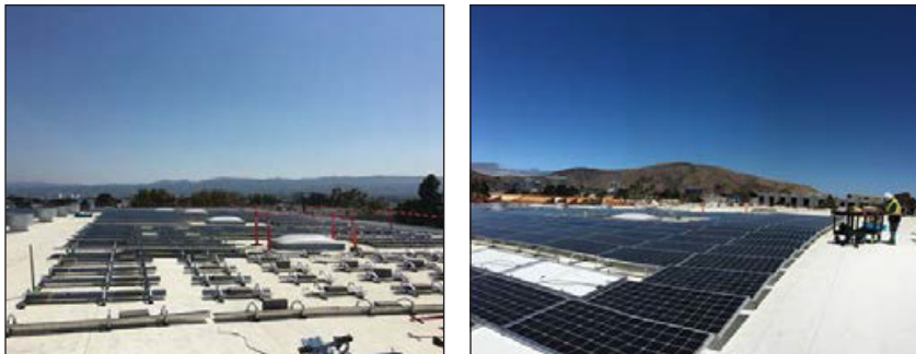
Solar Arrays atop Genentech Buildings
