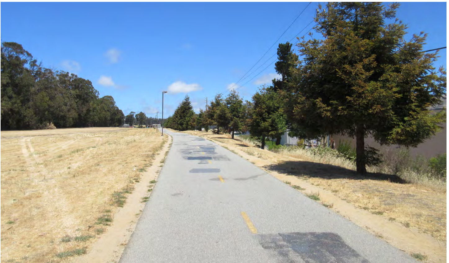
Site Photo - Image of typical trail section and current pavement condition.
