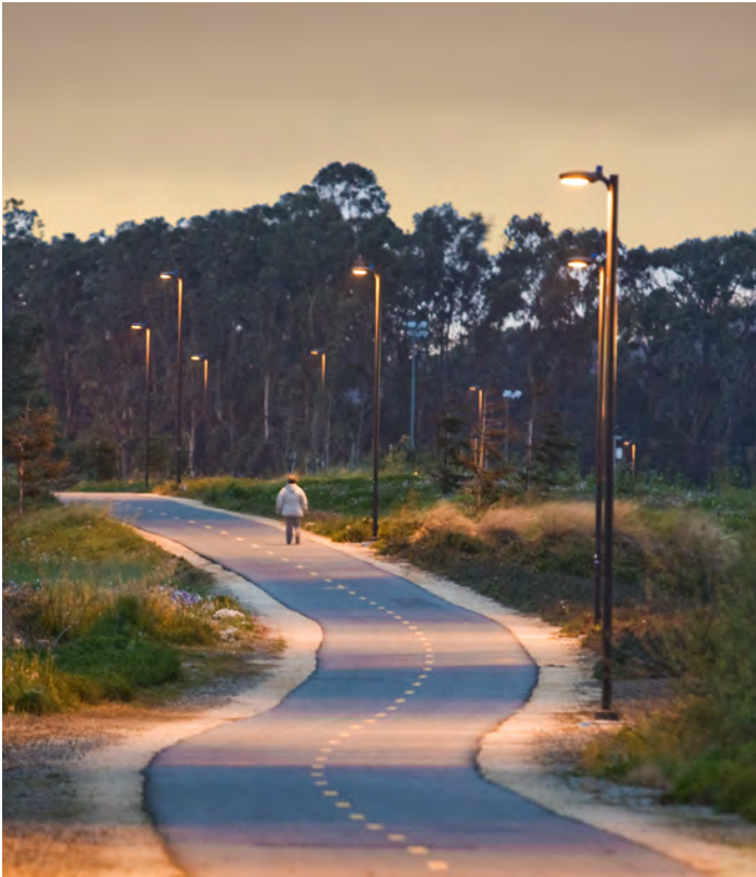
Site Photo - Trail lighting at dusk, taken shortly after construction.
