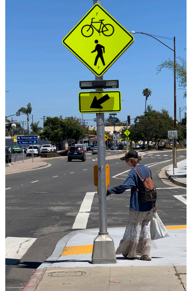
Rectangular Rapid Flashing Beacon (RRFB)
